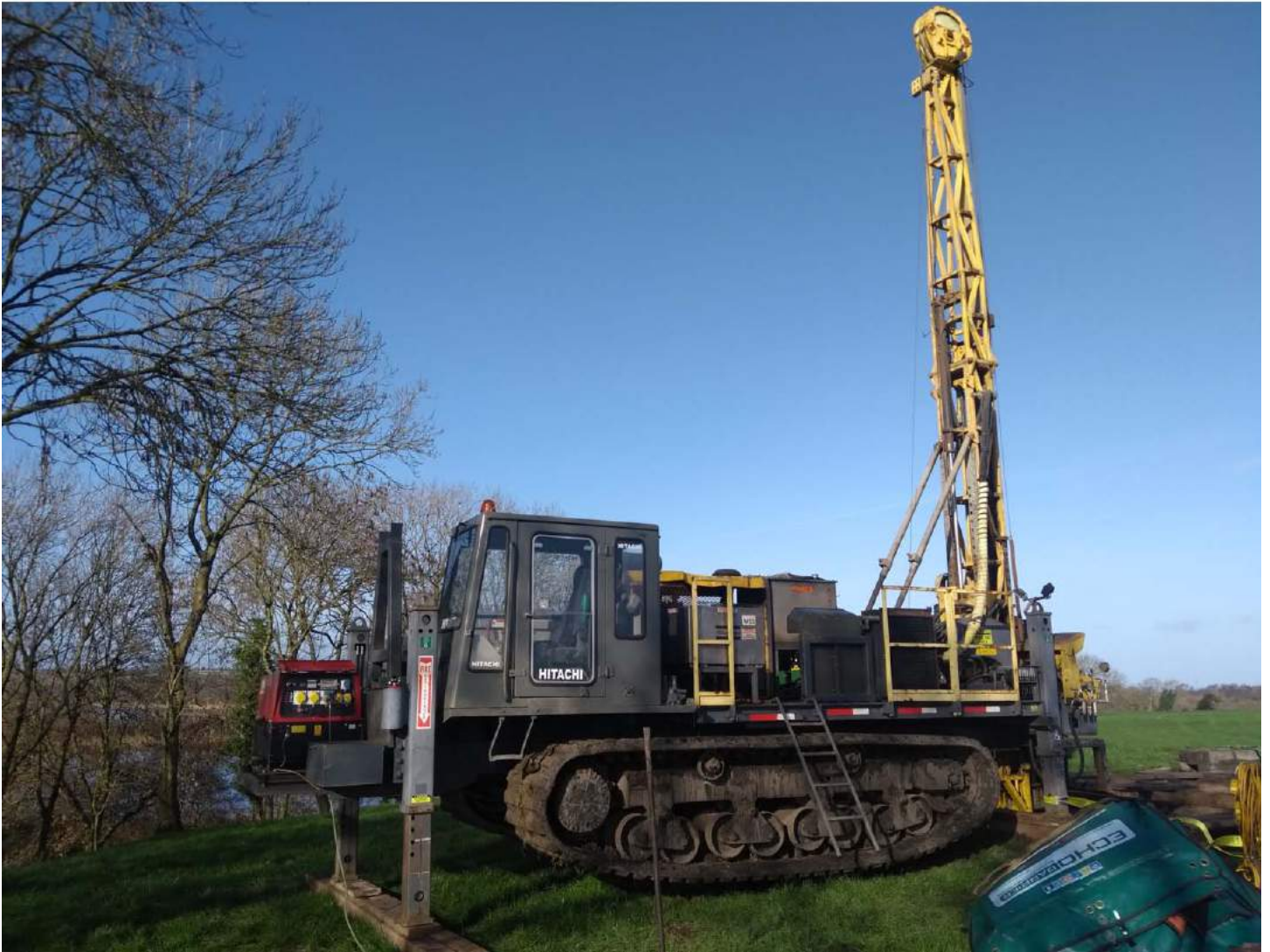
Photo 1: Drill rig sited over drill hole 11-3643-10 and ready to be extended by 200-250 metres to test the mineralized target zone at the base of the Waulsortian limestone. A lovely winter's day in Ireland!
